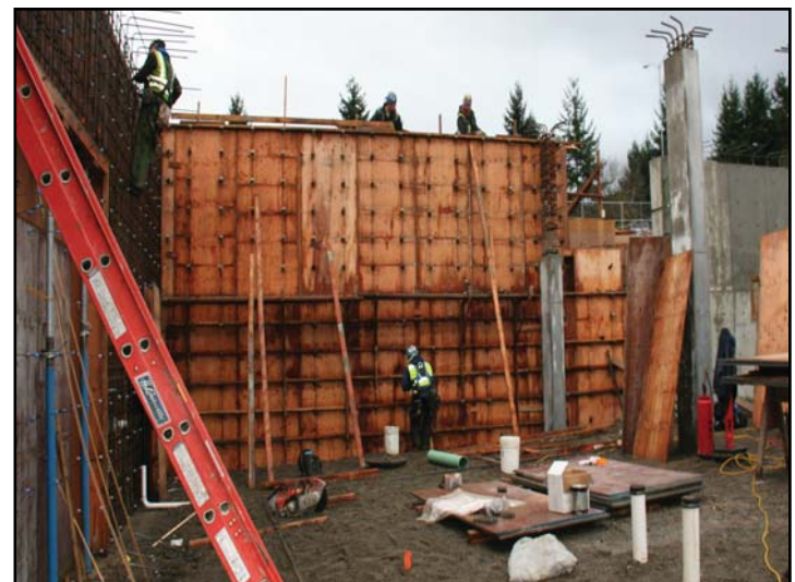
A work crew at Andrew's Glen forms walls on the northwest section of the building. Construction is on schedule to complete in Summer 2011.
