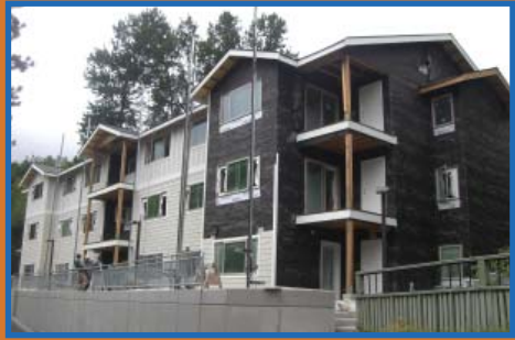
Johnson Hill Apartments in Issaquah is nearing completion. The new construction allows for eight new supported units in partnership with Hopelink.
